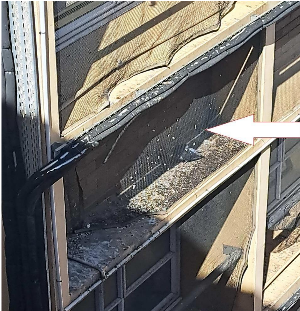
DAMAGED NET AND NEST REMOVAL
